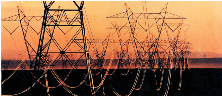
Transmission Line Conductors
